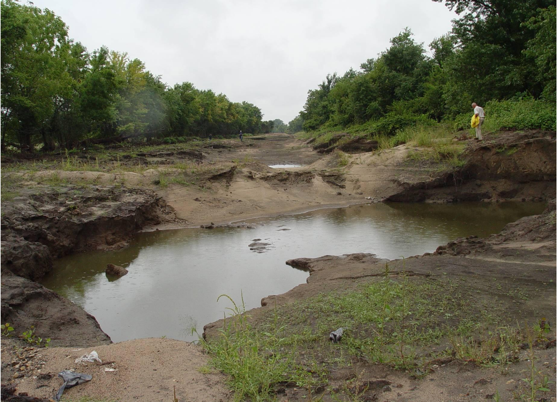
Scour holes in a shale foundation testified to a large volume of water sweeping through, leaving almost no trace of the levee behind
